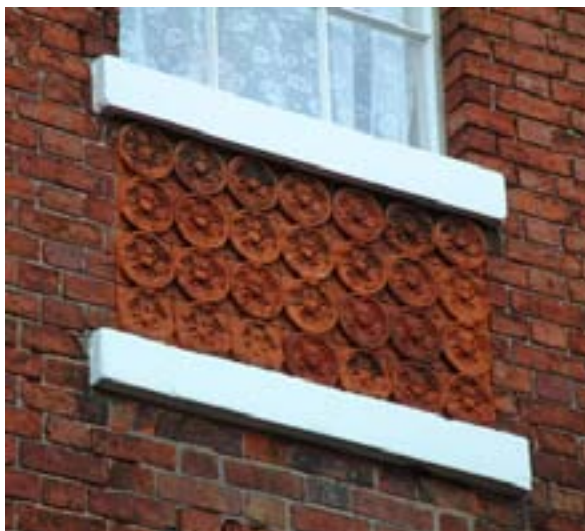
Below right - moulded red bricks used to create a roll-moulding for the window mullion and jambs. The same moulding continues in the stone lintel.
