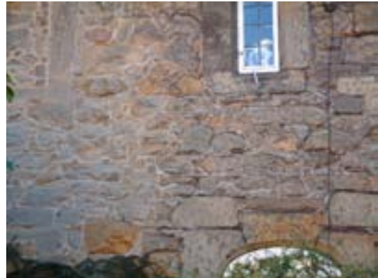
Above right - rubblestone with chamfered dressed window and door surrounds of the 17th century.
